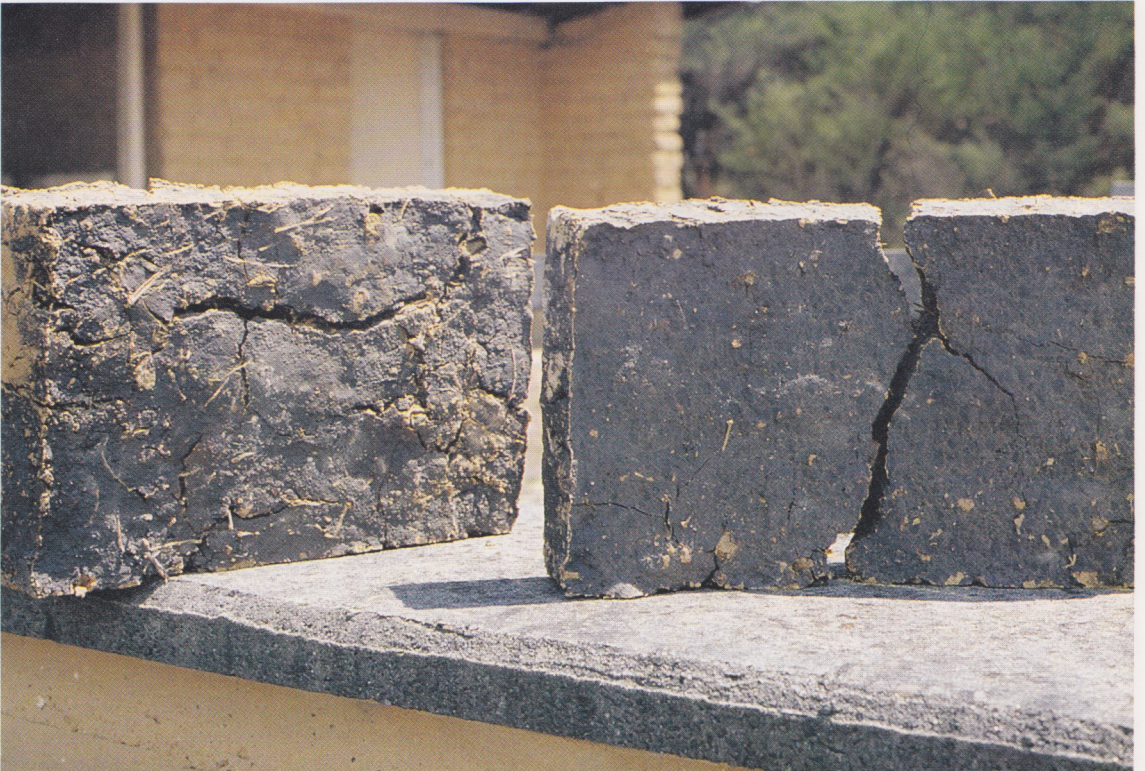
Fig. 5.2 – The use of straw in adobe blocks. Photograph (a) shows the appearance of adobe blocks one with too much straw and the other with the correct quantity of straw. Photograph (b) shows the crack-distributing effect of straw. Both the blocks were made from the same heavy clay, but the one without straw has cracked into two pieces.
